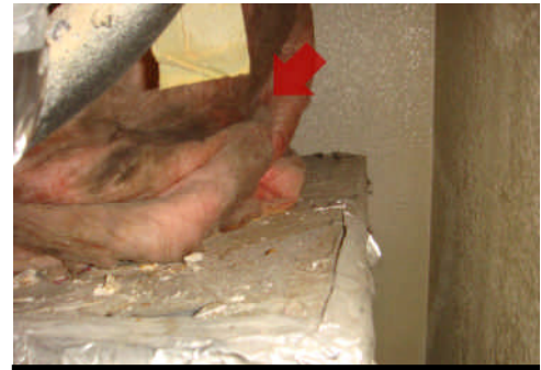
Suspected undersized supply plenum on coil
