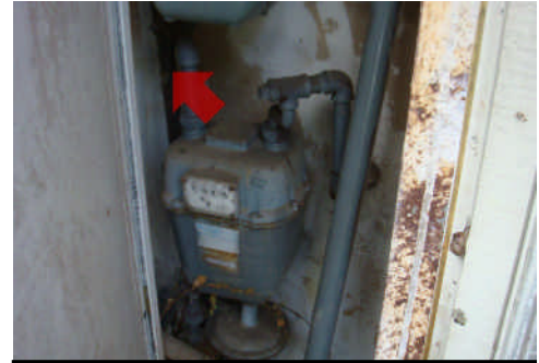
View of the gas meter. Valve is behind.
