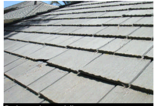
Broken and warped tiles.
