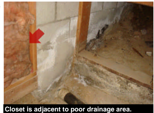
Closet is adjacent to poor drainage area.
