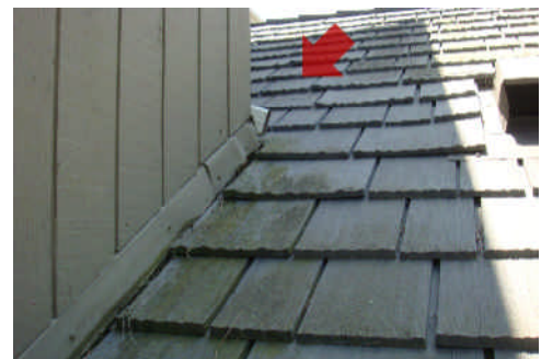
Back side chimney flashing not evaluated.
